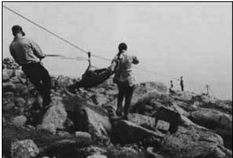
A loaded rock carrier has been lifted by the cable and is being moved to the Trail. Uphill worker (foreground) is using a spare strap to control the descent of the load. In this case, on the A.T. a half-mile from Baxter Peak, the carrier is a manual one with handles. We found it better to remove the handles and use two snatch blocks to center the load under the cable. (Photo by Lester C. Kenway)
